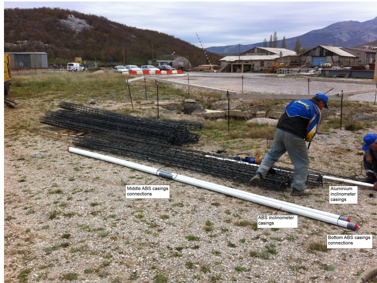
FIGURE 5.6: Six meter inclinometer ABS casings connected with ABS connection in the middle
