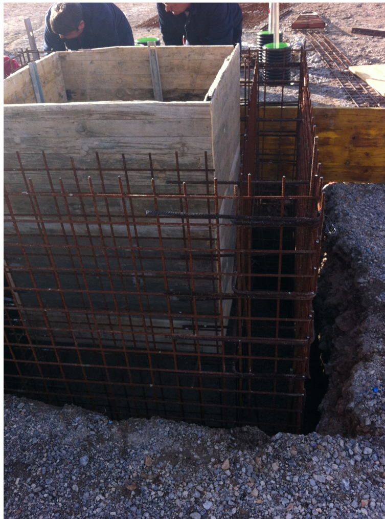
FIGURE 5.10: Counterweight block reinforcement
